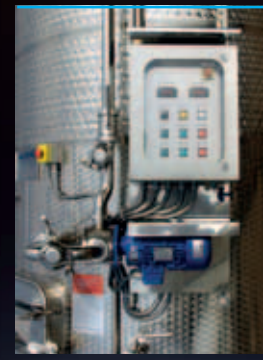
Electric board controlling the pump over pump or the punching down phases
