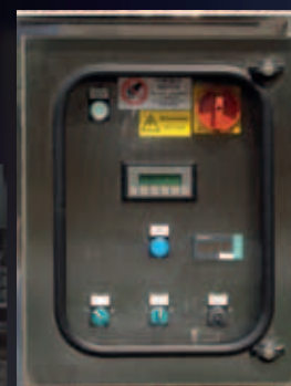
Control board for temperature and automatic pump over
